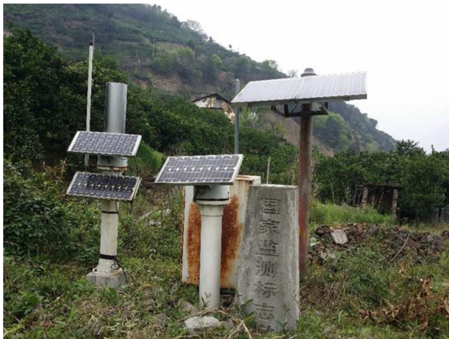
Fig. 3.5 Detecting rain gauge and deep deformation
