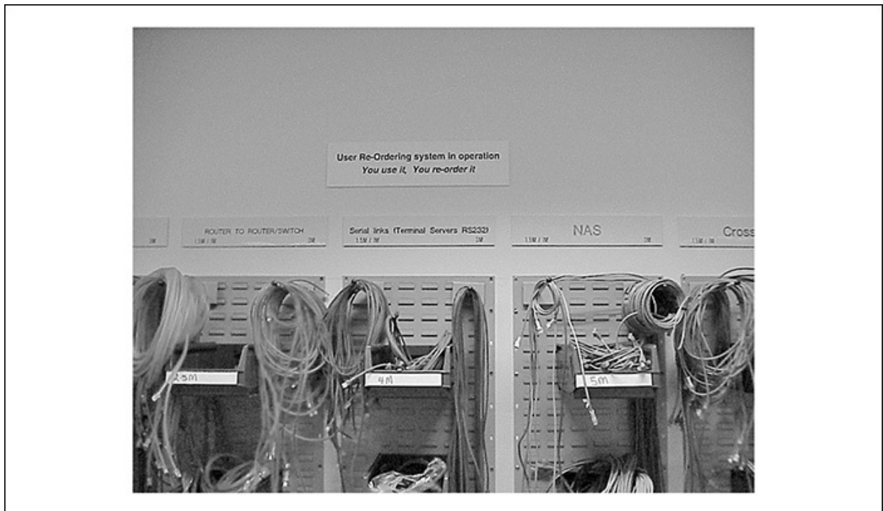
Figure 26.7: Blue bins and hanging cables at Eircom
